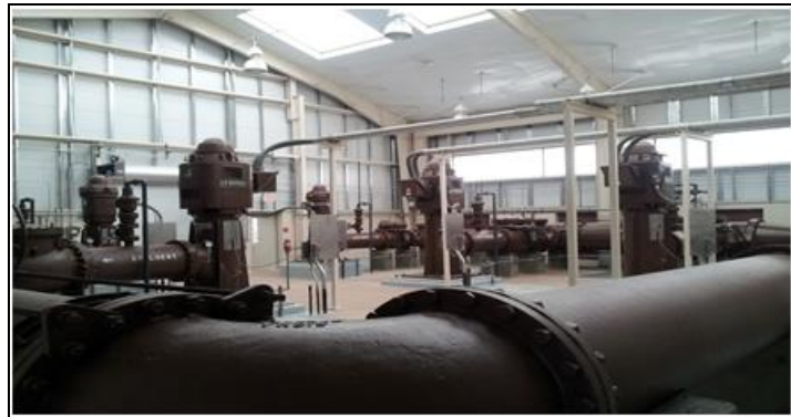
Figure 2-Effluent Pump Station Interior, Western Wake Regional Water Reclamation Facility
