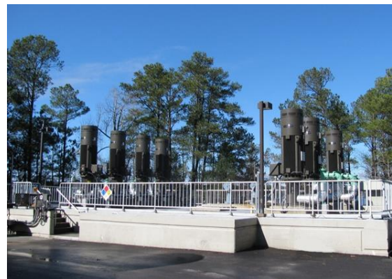
Figure 3- Jordan Lake Intake Pump Station
